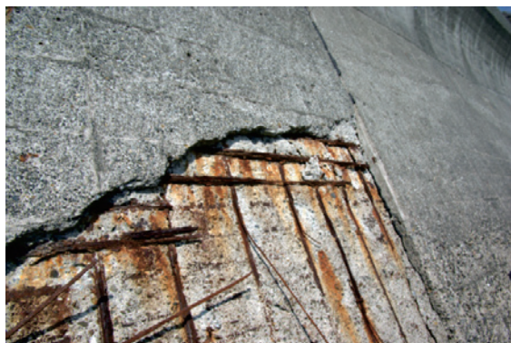
Fig.12 堤防の鉄筋の劣化（静岡県） Degradation of reinforcement bars in banks (Shizuoka prefecture)
