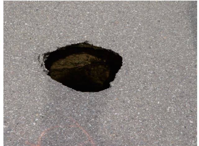
Fig.6 陥没の発生 (福井県) Occurrence of a cave-in (Fukui prefecture)
