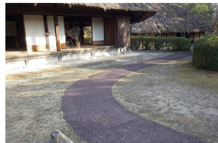
Fig.3 A promenade made of semi-carbonized pavement material that was experimentally constructed in a park in Yamatokoriyama City, Nara Prefecture (Provided by the Nara Forest Research Institute)
