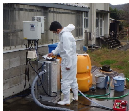
Fig.2 Installation and adjustment work for the BOD monitoring system at the Tottori Swine & Poultry Experiment Station (Provided by DKK-TOA Yamagata Corporation)
