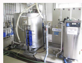
Pre-Cooling system for raw-milk using a CO 2 heat pump.
