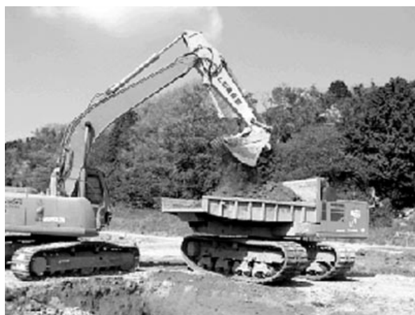
Fig.14 バケット式解砕機による解砕状況 Crushing of initial-stabilized soil by bucket-type crusher machine
