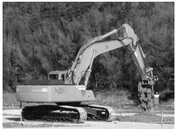
Fig.12 トレンチャーによる初期固化状況 Initial stabilization of muddy soil by trencher-type mixing machine
