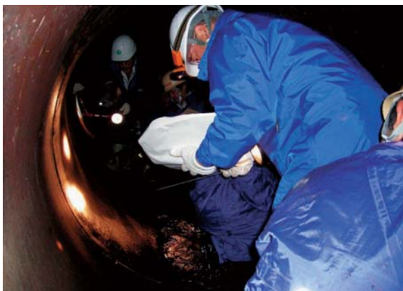
■ Inspection of main pipeline damaged by the Iwate-Miyagi Inland Earthquake in 2008
