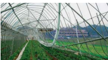
■ Gathering data on greenhouses damaged by disasters for structural analysis
