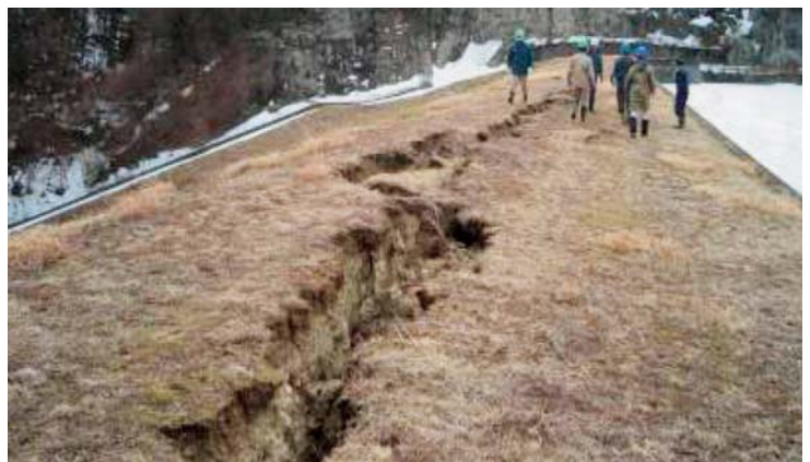
■ Hazard assessment of a reservoir embankment damaged by the East Japan Earthquake Disaster in 2011
