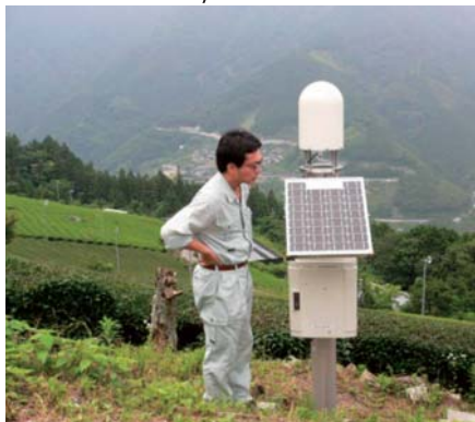
■ GPS landslide-displacement observation system
