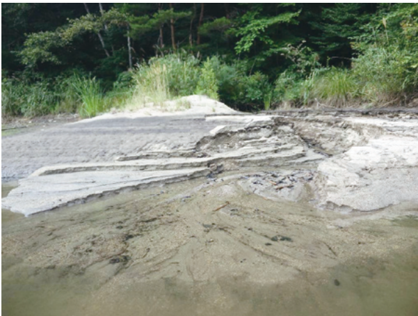
Fig.12 ため池流入部の底質の浸食状況 (9月11日) Bottom sediment in part of the reservoir inflow (2013/9/11)
