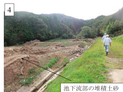
Fig. 24 ⑦池下流部の堆積土砂 Deposited sand at downstream part of ⑦ ike
