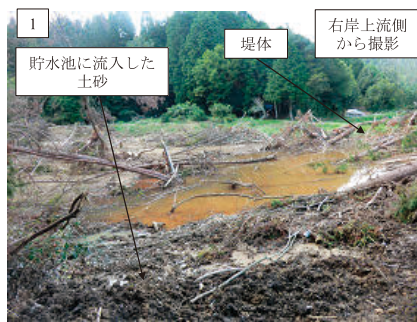
Fig. 26 ⑧池貯水池内の堆積土砂 Deposited sand of ⑧ ike
