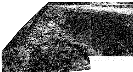
Photo 1 浅い円弧滑りによる法面崩壊 (Fig. 5のA) Slope failure by shallow slip circle
