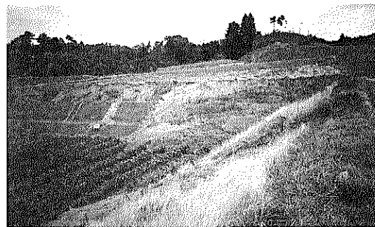
Photo 15 No.2 (遠方) 及びNo.3 (手前) の法面崩壊 Slope failure at No.2(distance) and No.3(near) slope
