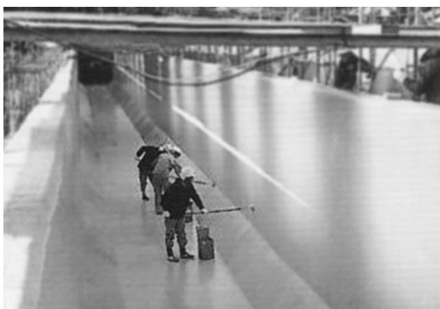
Fig.10 表面被覆工法（塗装工法）の例 Concrete surface protection method (painting method)
