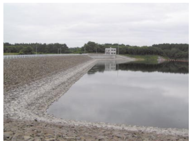
Fig.19 宿の沢ダムの改修後の堤体上流側の状況 Upstream view of Syukunosawa dam
