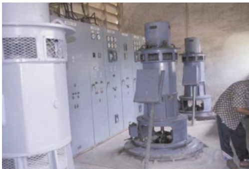
Fig.31-2 揚水機場ポンプ Pumps in the pumping station
