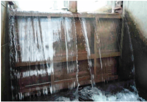
Fig.17 水膜の発生状況 Current state of water screen
