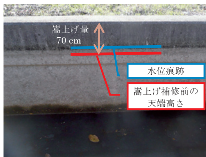
Fig.17 嵩上げ補修最大時（嵩上げ量 70cm） の水位痕跡と補修前の天端高さの比較 Comparison between water level trace and previous wall edge height in the maximum expansion situation
