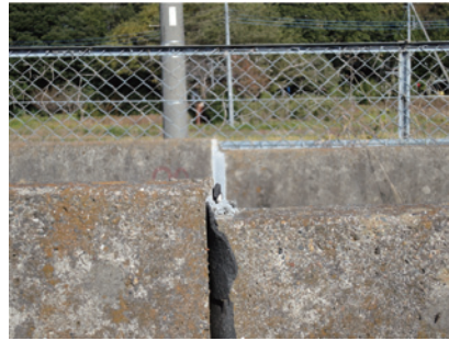
Fig.10 台通用水路 下流未改修区間のバレル間の不同沈下 Subsidence between the barrels of the downstream non-repair section
