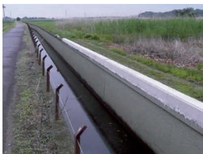
Fig.16 溢水が生じた区間の嵩上げ補修状況 The expansion of canals walls on the section where overflow occurred
