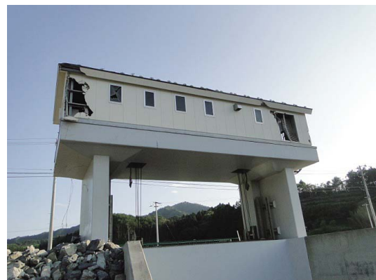
Fig. 85 操作室外壁の破損 Damage of external wall of control room
