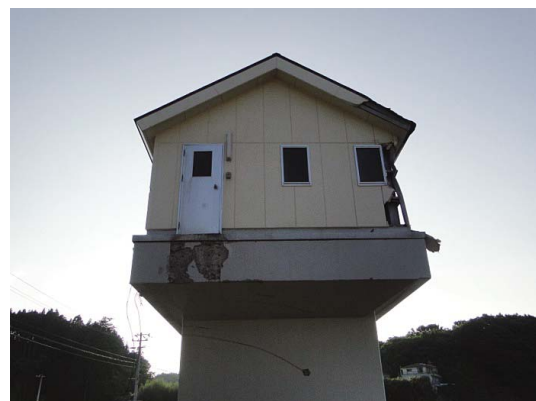
Fig. 86 操作室の取り付け階段の喪失 Loss of mounting stairs toward the control room
