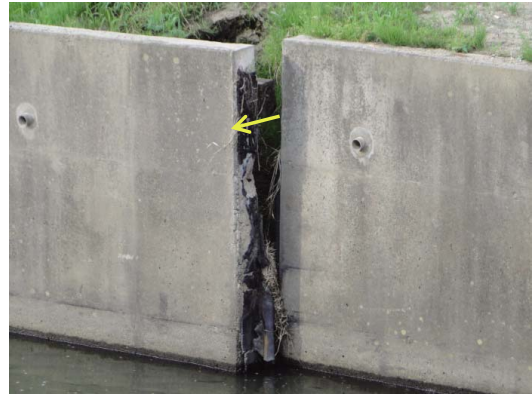
Fig. 44 堰下流右岸擁壁の変位 Lateral displacement of retaining wall
