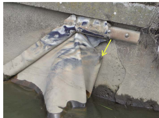
Fig. 2 ゴム堰袋体の端部の破断 Broken end of rubber tube
