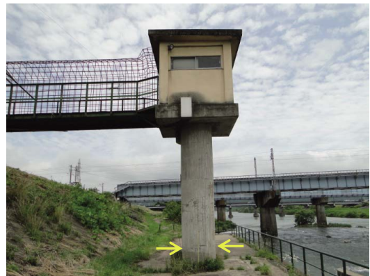
Fig. 56 操作室の柱基部にひび割れ Crack at the base of the pillar of the control room
