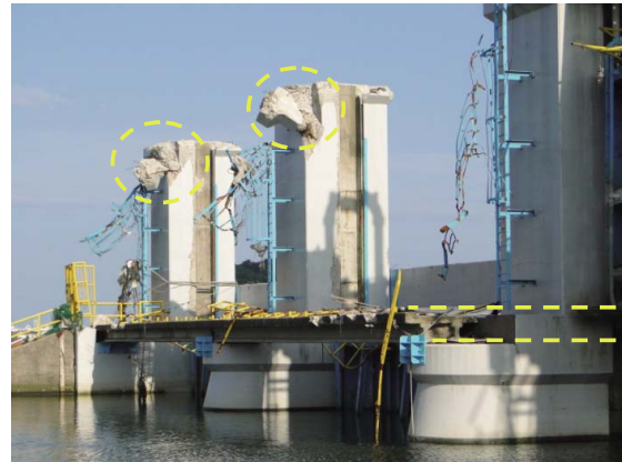
Fig. 6 上部管理橋の落橋に伴う門柱上部の損傷 Damage to the top of gatepost caused by dropped bridge
