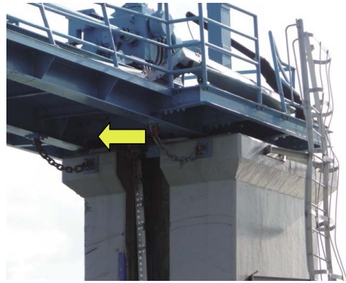
Fig. 72 上部管理橋が海側へ桁ずれ Displacement toward sea side of upper maintenance bridge
