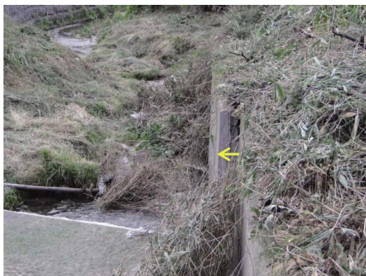
Fig. 49 下流右岸擁壁の押し出し Lateral displacement of retaining wall
