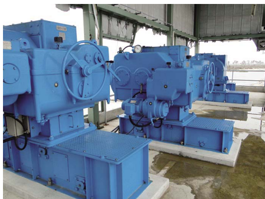
Fig. 99 開閉装置の状態 Gate opening and closing apparatus
