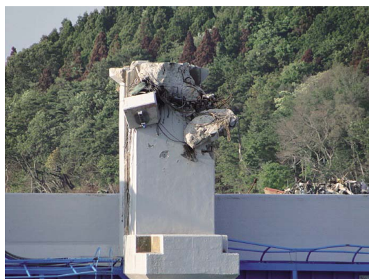
Fig. 83 門柱上部の損傷 Damage to the top of the gatepost
