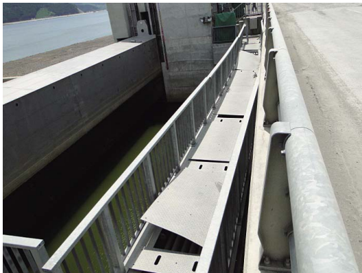
Fig. 88 下部管理橋の変形 Deformation of the lower maintenance bridge
