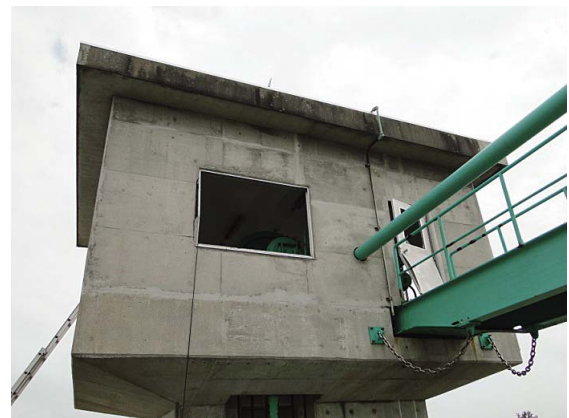
Fig. 12 機側操作室の窓およびドアの破損 Damage of the window and door of control room
