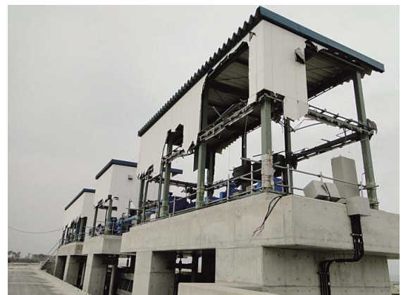
Fig. 11 機側操作室外壁の破損 Broken wall of control room
