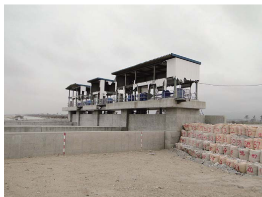
Fig. 98 操作室外壁の破損 (海側) Broken wall of machine room
