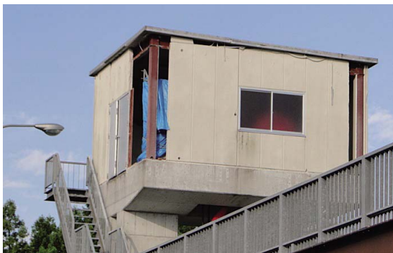
Fig. 24 操作室の外壁パネル脱落状況 Falling of external wall panels of control room
