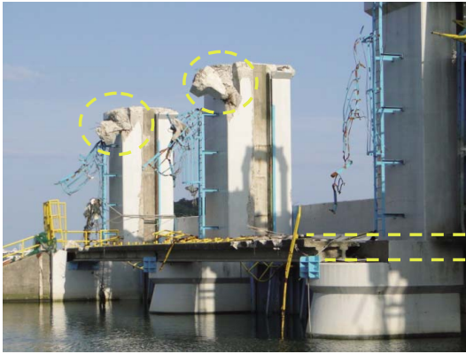
Fig. 75 上部管理橋の落橋に伴う門柱上部の損傷 Damage to the top of gatepost caused by dropped bridge
