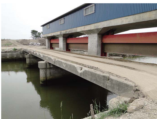
Fig. 101 管理橋欄干の破損 Damage of balustrade of maintenance bridge
