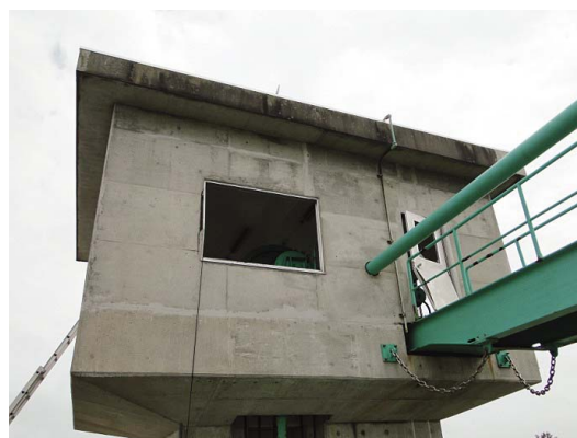
Fig. 103 操作室のドアおよび窓の破損 Damage of the window and door of control room
