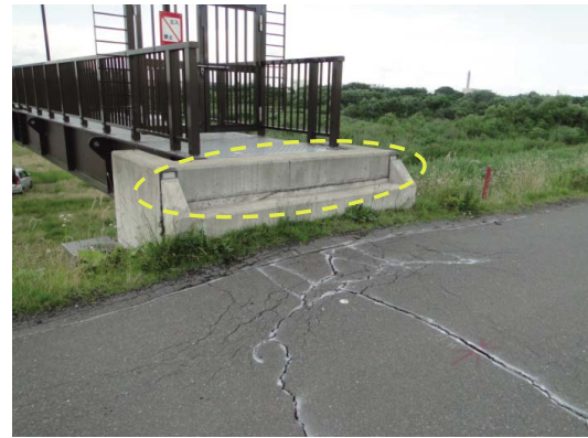
Fig. 31 堤防の沈下による管理橋取り付け部の段差 Difference in level at the junction with maintenance bridge caused by bank subsidence
