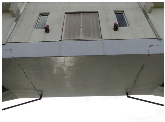
Fig. 92 中央径間の操作台下部の両側にひび割れ Cracks on both sides under the operation unit of the center span
