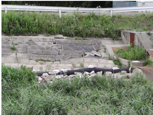
Fig. 41 堰下流右岸の護岸ブロックの崩れ Collapse of bank protection blocks at the right bank
