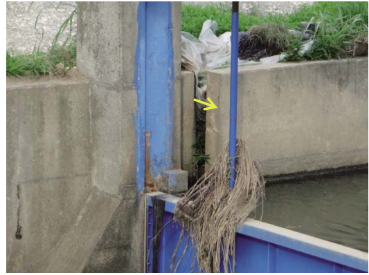
Fig. 43 堰上流右岸擁壁の変位 Lateral displacement of retaining wall
