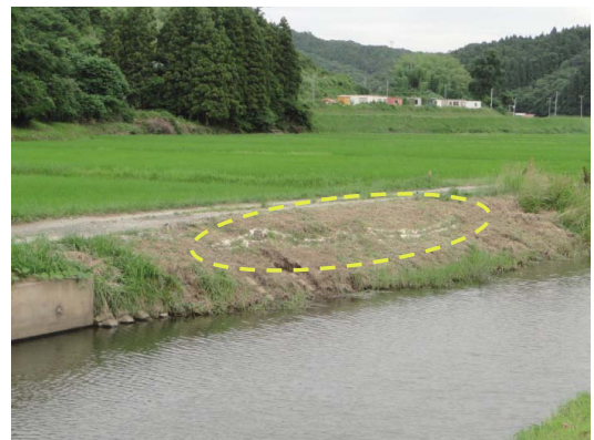
Fig. 45 法面のすべり Landslide on a right bank slope
