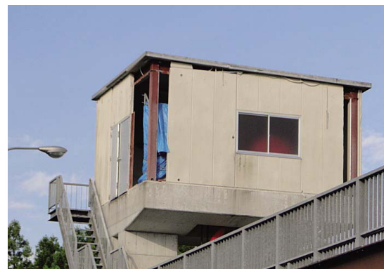
Fig. 3 外壁パネル脱落状況 Falling of external wall panels of control room
