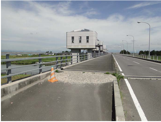
Fig. 34 管理橋に生じた段差 Difference in level at the junction with maintenance bridge
