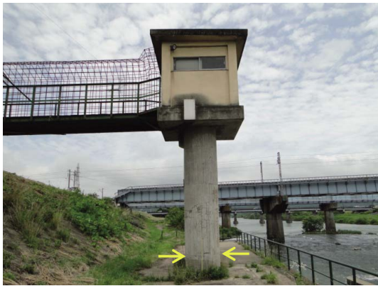
Fig. 4 操作室の柱基部にひび割れ Crack at the base of the pillar of the control room
