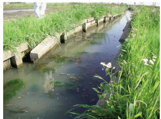
Fig. 71 柵渠の沈下・傾き（北割排水機付近）（地点番号 3） Settlements and inclination of the concrete pile canals (around the Kitawari pumping station) (No.3)
