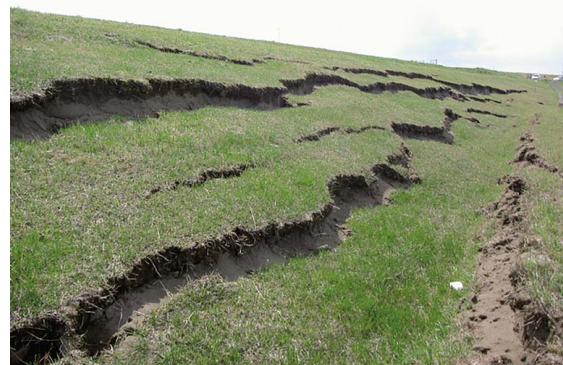
Fig. 49 堤防法面の亀裂 (川裏) Cracks on the slope of the bank (on the side of the landward)
