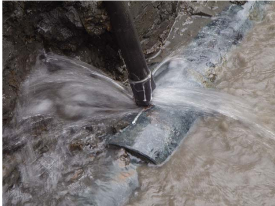
Fig. 79 枝管への分岐部での漏水 Water leakage at the joint of branch pipe
