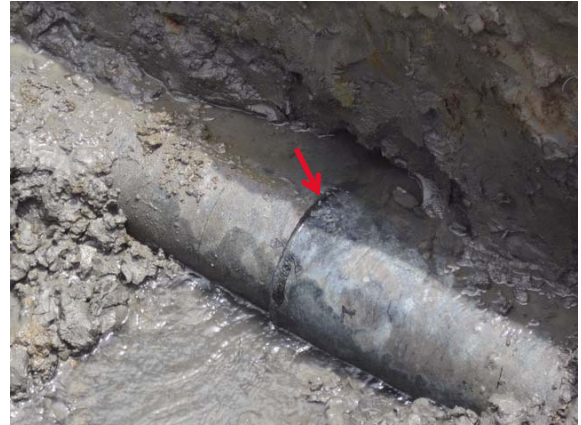
Fig. 81 石綿管のせん断破壊 Shear failure of an asbestos pipe
