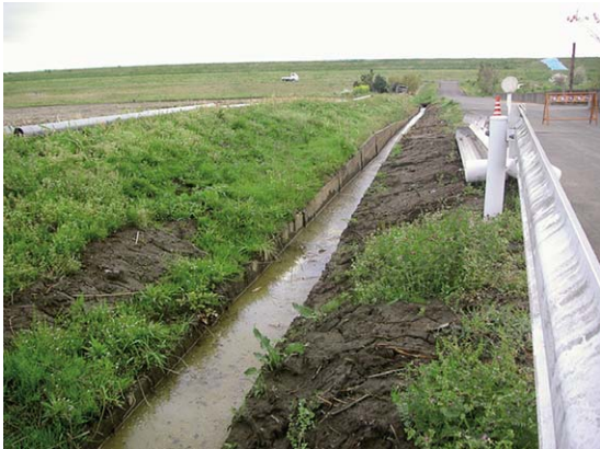
Fig. 45 排水路の浮上 Uplift of drainages
