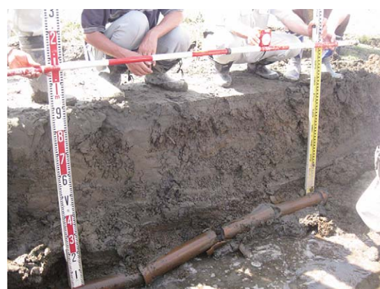
Fig. 24 陶製暗渠管の不陸と継手での損傷 Unevenness and damages of joints of unglazed drain pipes
