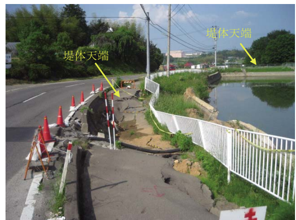
Fig. 35 田桑池左岸池敷の道路の崩落 Failure of a road along the reservoir of Takuwa dam
