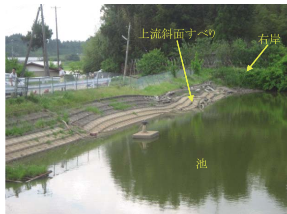
Fig. 30 北の内ため池上流斜面のすべり Sliding on the upstream slope of Kitanouchi dam
