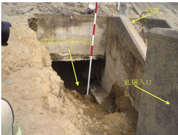
Fig. 33 底樋入口左岸側の堤体土の吸出し Erosion of the upstream slope into the cracked inlet pipe dam
