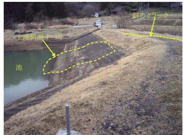
Fig. 20 細蕨ため池の被災状況 Condition of Hosowarabi dam after the earthquake
