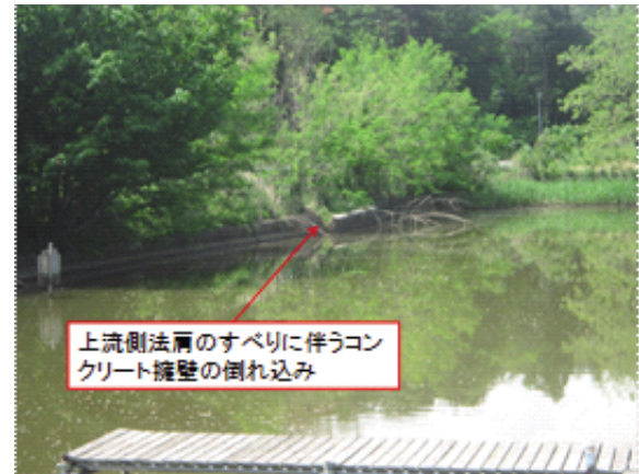
Fig. 29 菖蒲池上流斜面波除工の転倒 Falls of erosion-protection walls on the upstream slope of Shobu dam
