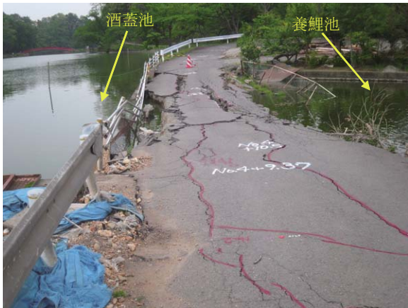
Fig. 23 酒蓋池と養鯉池との境界部の崩落 Failure between Sakabuta dam and a neighbored fishery pond
