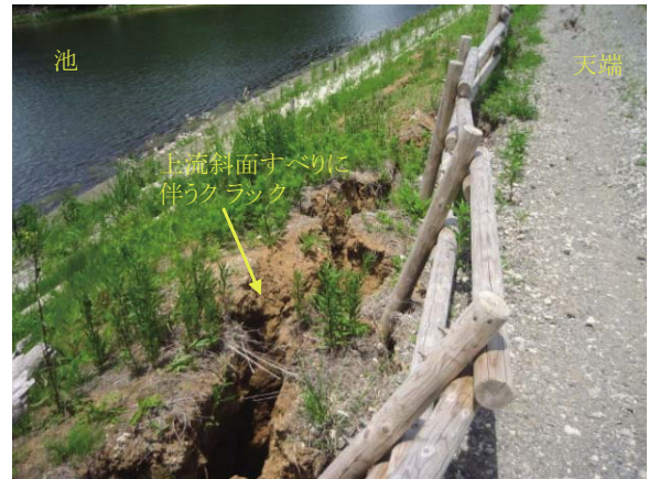
Fig. 38 笹平池上流斜面の崩落 Sliding on the upstream slope of Sasadaira dam
