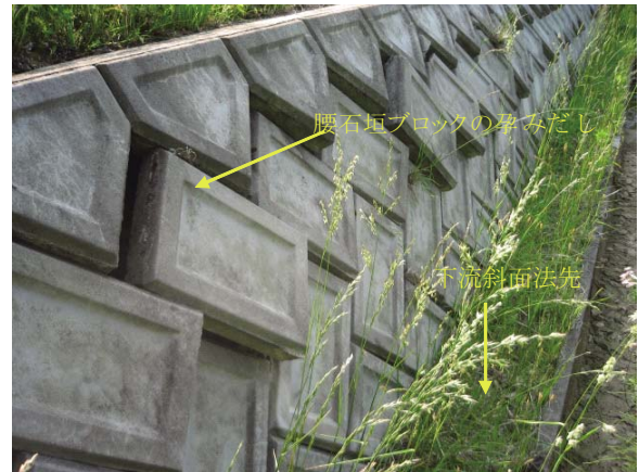
Fig. 34 田桑池の腰石垣の孕み出し Deformation of toe drain blocks of Takuwa dam
