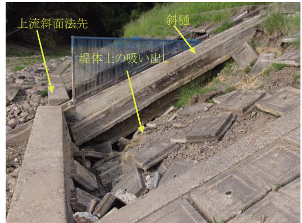
Fig. 25 二池底樋入り口周辺の吸い出し Erosion around the entrance of the outlet pipe at Futaike dam
