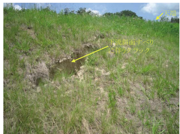
Fig. 39 笹平池下流斜面のクラック Longitudinal cracks on the downstream slope of Sasadaira dam
