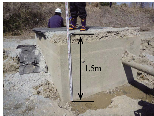
Fig. 36 矢吹南第 2 空気弁工の浮上 Uplift of Yabukiminami No.2 air valve
