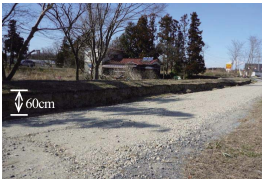
Fig. 50 バイプライン敷設道路の沈下 (大池西合流工周辺) Settlement of the road above a pipeline around OikeNishi confluent structures
