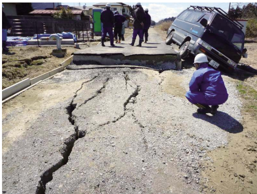
Fig. 40 パイプ敷設道路の亀裂 (矢吹第3・4 幹線分水工周辺) Cracks on the road around Yabuki No.3・4 division works of main pipeline
