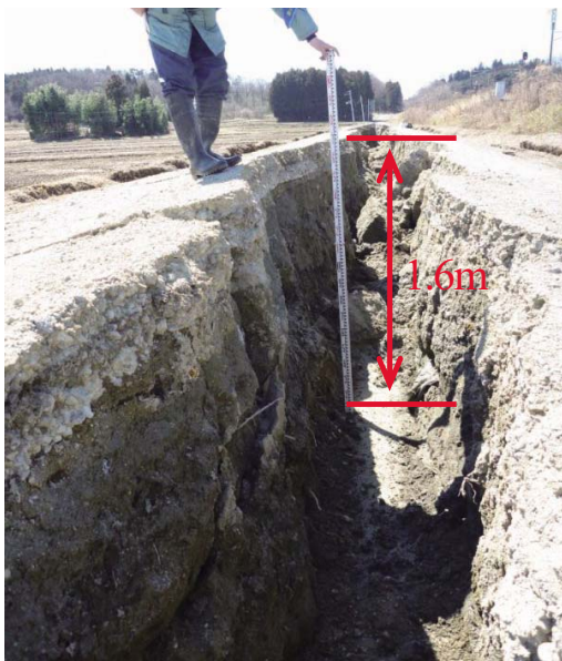
Fig. 35 パイプ敷設道路の亀裂 (矢吹南第 2 空気弁工) Cracks on the road around Yabukiminami No.2 air valve
