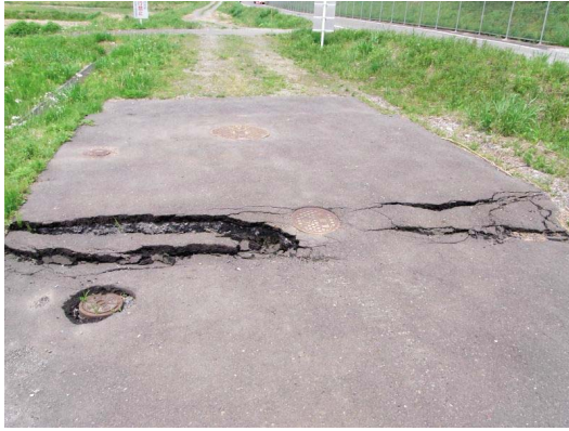
Fig. 28 五本松第3分水工の路面亀裂 Cracks on the road at Gohonmatsu No.3 division works
