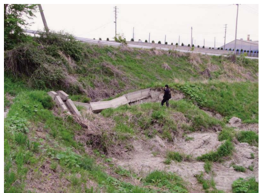
Fig. 23 信夫第3排泥工周辺の斜面崩壊 Slope failure around Shinobu No.3 blow off
