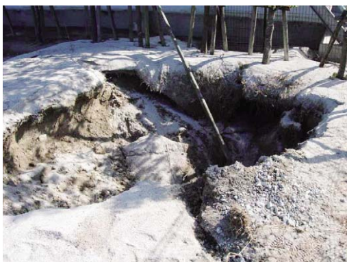
Fig. 53 管の離脱 (大池西合流工周辺) Separation of a pipe around OikeNishi confluent structures
