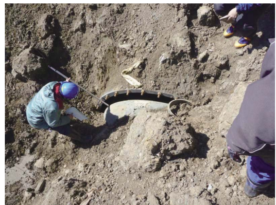
Fig. 26 五本松第1分水工周辺の片落管の離脱 Separation of a reducer around Gohonmatsu No.1 division works
