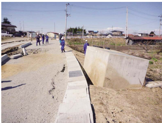
Fig. 46 矢吹北第 5 排泥工の浮上 Uplift of Yabukikita No.5 blow off
