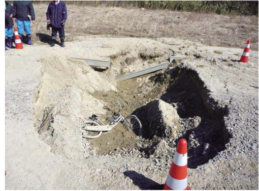
Fig. 47 片落管の離脱 Separation of a reducer
