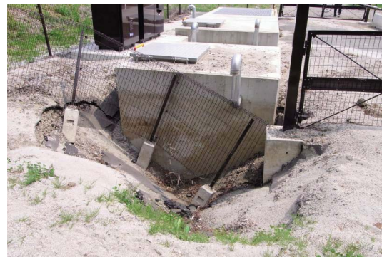
Fig. 31 矢吹南第2幹線分水工の路面陥没 Cave-in in the road surface at Yabukiminami No.2 division works
