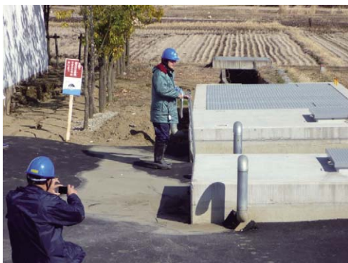
Fig. 52 構造物周辺の路面沈下 (大池西合流工周辺) Settlement of the road around OikeNishi confluent structures
