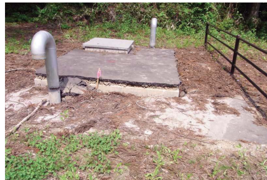
Fig. 30 矢吹南第1空気弁工の浮上 Uplift of Yabukiminami No.1 air valve
