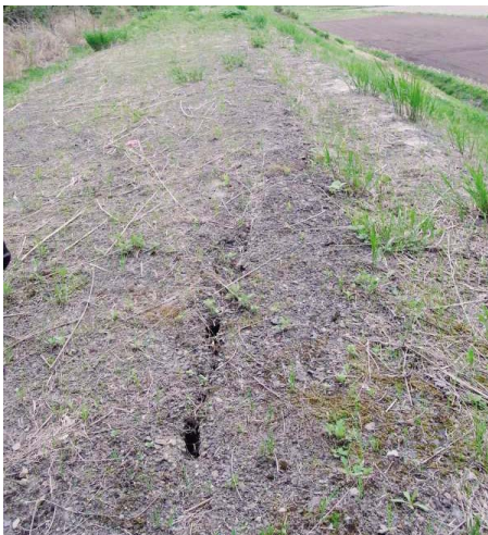
Fig. 18 パイプ敷設道路の亀裂 (信夫第7空気弁工周辺) Cracks on the road above a pipeline around Shinobu No.7 air valve
