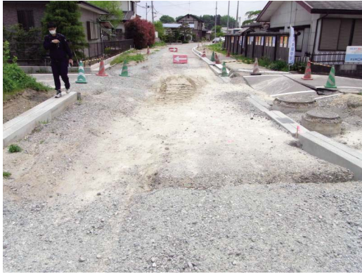
Fig. 44 矢吹北第 4 排泥工の路面の沈下 Settlement of road surface around Yabukikita No.4 blow off
