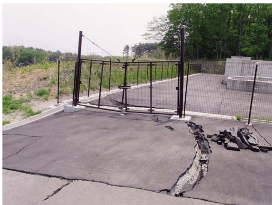
Fig. 24 踏瀬調圧水槽 Fumase surge tank
