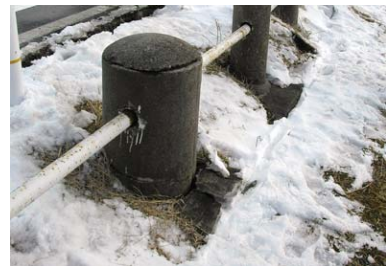
(c) 旧高欄の沈下と基礎破損
