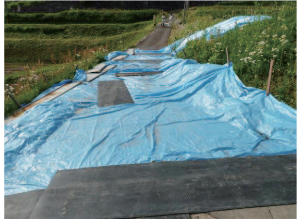
Fig. 16 農道の損傷箇所の応急対策 Emergency measures of damaged road
