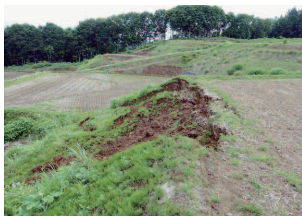
Fig. 12 畦畔法面の崩壊 Collapse of a levee slope
