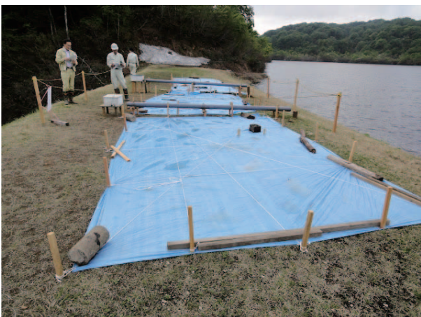
Fig. 37 堤頂部亀裂の観測状況 Observation of cracks on the top of embankment
