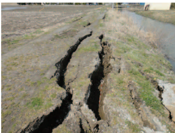
Fig. 22 農道の被害 Damage of farm road
