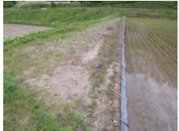
Fig. 19 仮畦畔の設置（能登半島地震） Installation of the temporary levee (Noto Hanto Earthquake in 2007)
