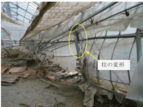
Fig. 21 津波の被害を受けた大屋根型連棟温室 (①) の内部の状況 Internal situation of damaged multi-span greenhouse (No. 1) by the tsunami
