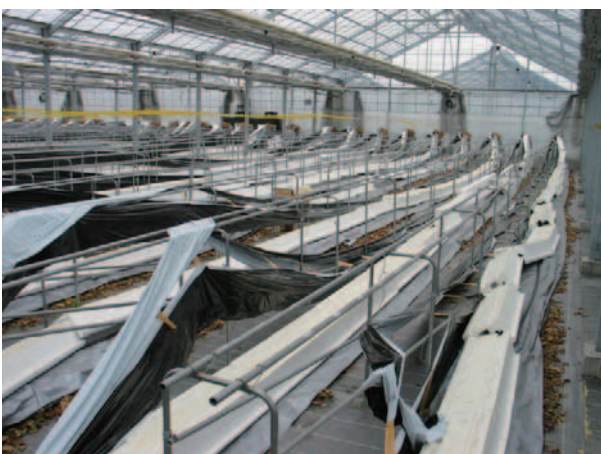
Fig. 38 地震動の被害を受けた高設栽培ベッドの状況 Situation of damaged high bench cultivation system by seismic motion
