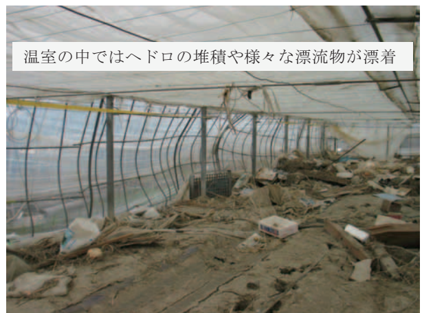
Fig. 24 津波の被害を受けた大屋根型連棟温室 (②) の内部の状況 Internal situation of damaged multi-span greenhouse (No. 2) by the tsunami
