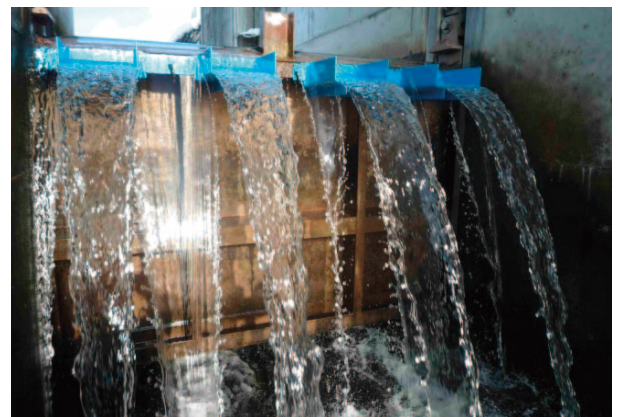
Fig.20 対策工からの越流状況 Overflow state through countermeasure works
