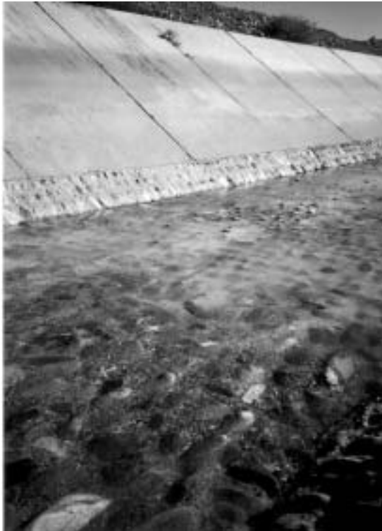
Fig. 46 A Lining of the Changma Old Main Canal at an area with a steep-slope in Gansu Province. (September, 1995)
