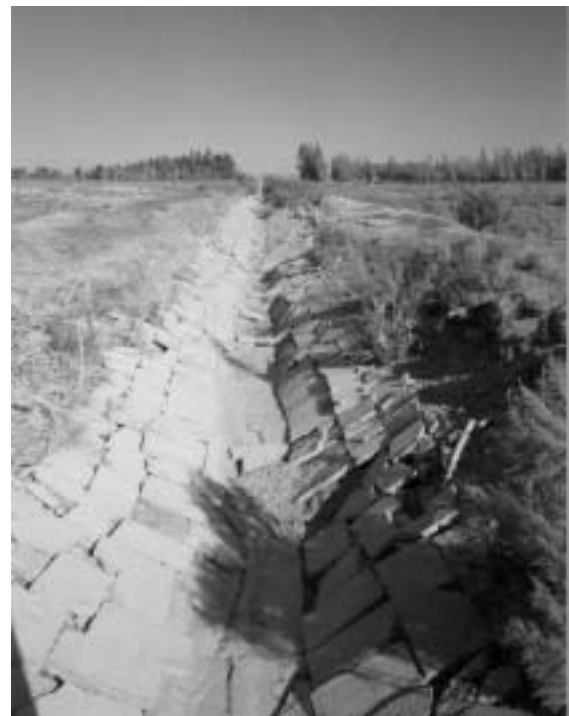
Fig. 41 Canal Seriously Damaged by Freezing in Gansu Province. (October, 1995)
