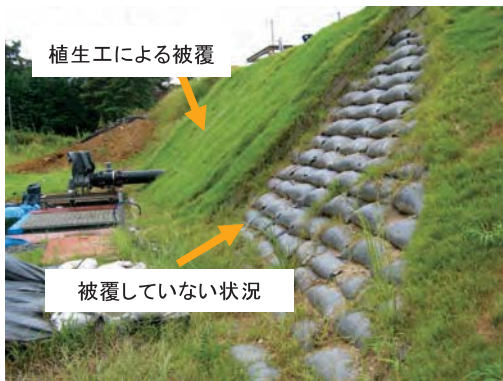
Fig. 267 土嚢積層斜面の植生工による土嚢材の紫外線劣化対策 Protection of slope surface by plant cover to prevent ultraviolet ray degradation
