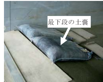
Fig. 187 所定の角度で整形した基盤面と土嚢の設置状況 Inclined base arranged at prescribed angle and installation of soil bags
