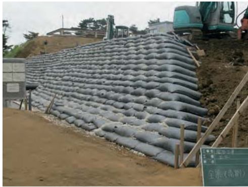
Fig. 266 所定の段数まで土嚢を積み上げた状況 Completion of stacking geosynthetic soil bags up to prescribed steps
