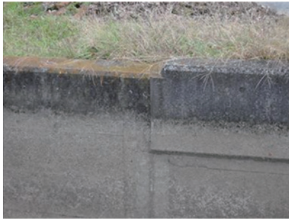
Fig.9 改修区間(左)と未改修区間(右)の境目 Border of repair section (left) and non-repair section (right)
