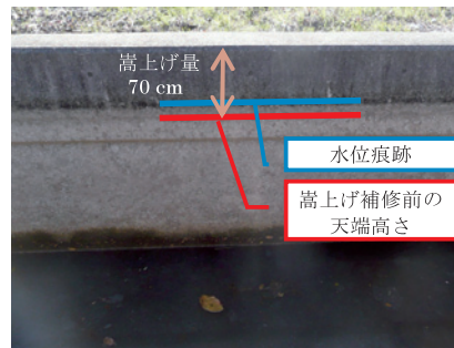
Fig.17 嵩上げ補修最大時（嵩上げ量 70cm） の水位痕跡と補修前の天端高さの比較 Comparison between water level trace and previous wall edge height in the maximum expansion situation
