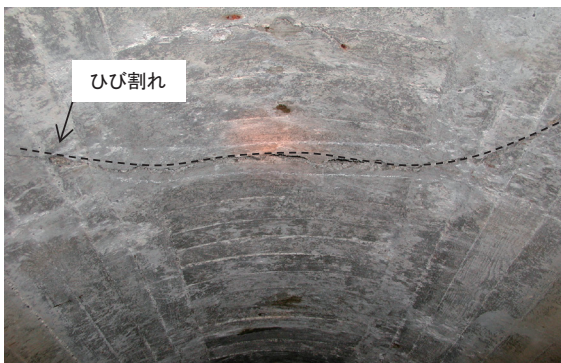
Fig.9 押し抜きせん断破壊 Shear failure in the crown
