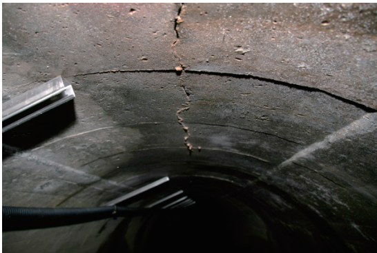
Fig.7 天端部のひび割れ Cracks in the crown
