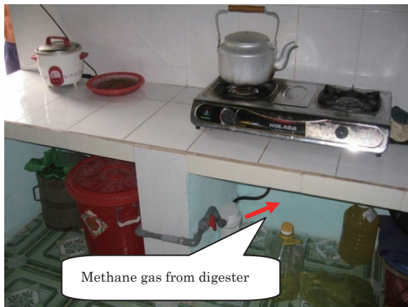
(c) Utilization of biogas in a kitchen
