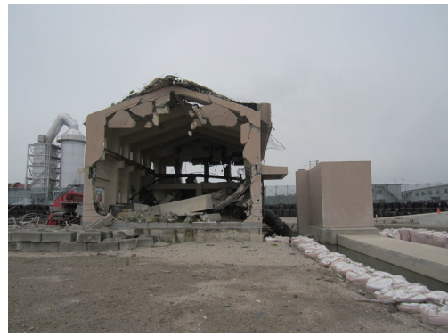
Fig.5 排水機場の津波による被災状況 Damage to a drainage pump station caused by the tsunami
