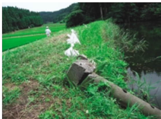
Fig.15 斜樋の損傷 Damage to inlet works
