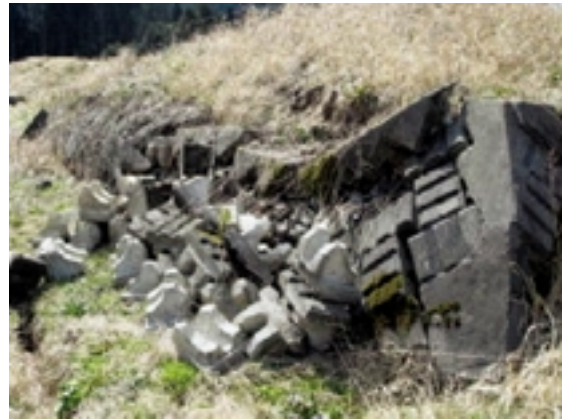
Fig.20 擁壁の崩壊 Close-up of retaining wall failure
