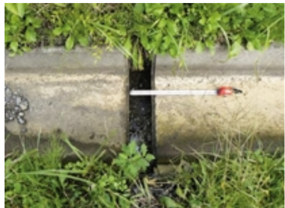
Fig.39 目地のずれ Separation of a canal joint
