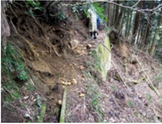
Fig.2 用水路への土砂流入 Inflow of earth and sand into an irrigation canal
