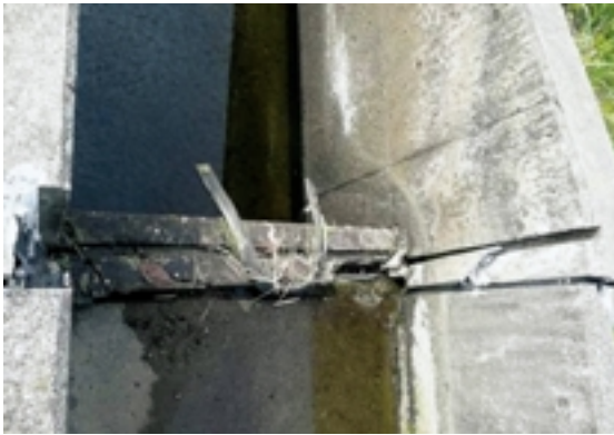
Fig.23 目地付近角落としの倒壊 Collapse of sliding timber at a canal joint
