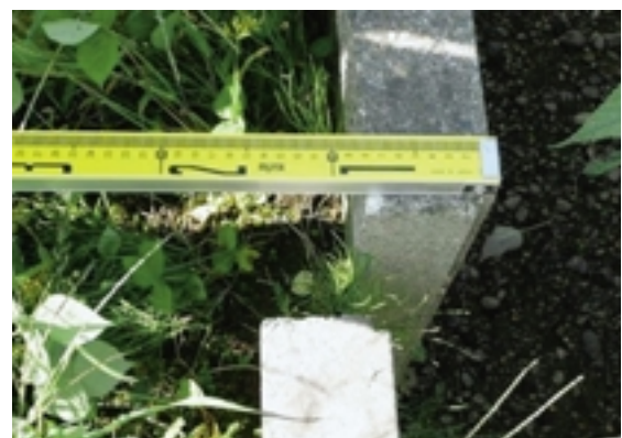
Fig.16 排水フリウムにおける目地のずれ Offsetting of the joint of a drainage flume
