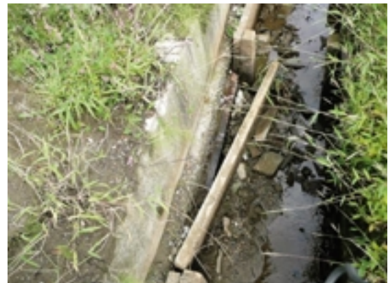
Fig.50 コンクリート柵渠柵板の崩落 Breakage and collapse of fence boards in a concrete drainage canal
