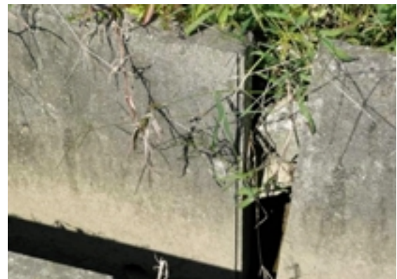
Fig.15 排水フリウムにおける目地の開き Expansion at a joint in a drainage flume
