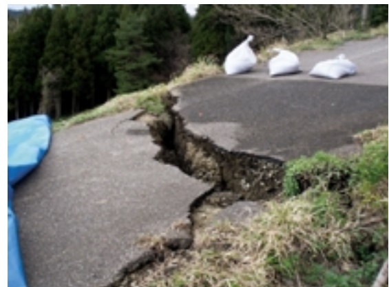
Fig.6 農道の亀裂 Fissure on a farm road
