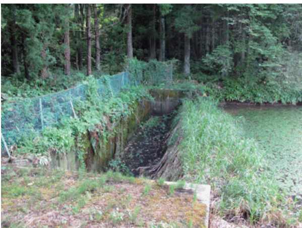
Fig.2-5 洪水吐流入口付近に繁茂する雑草 The weed which grows thick in front of spillway
